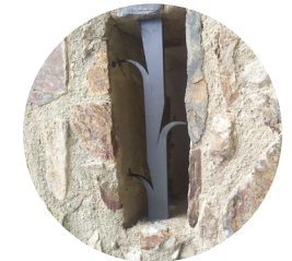
Window and estripagec (metal bars with irregular lateral spikes placed at windows to stop anyone entering)
